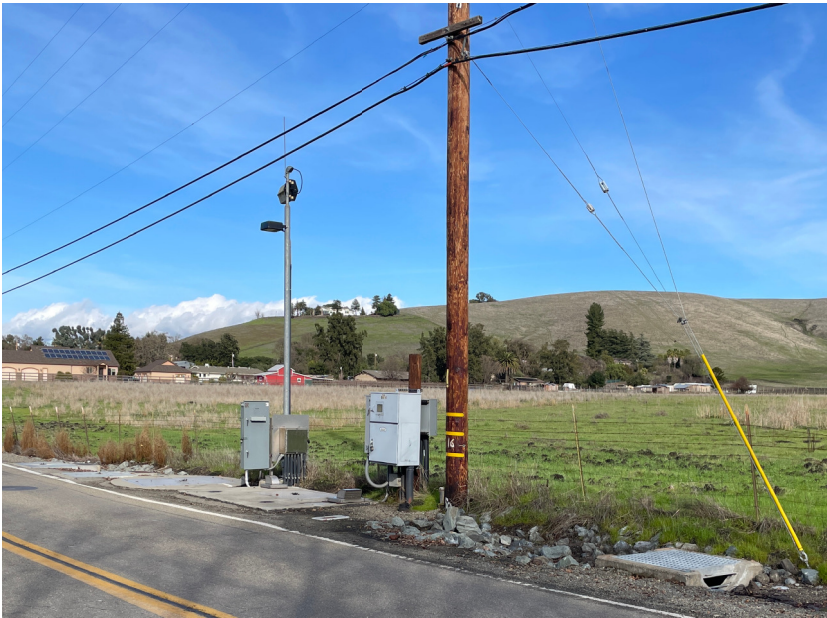
EXISTING LIFT STATION PHOTO
