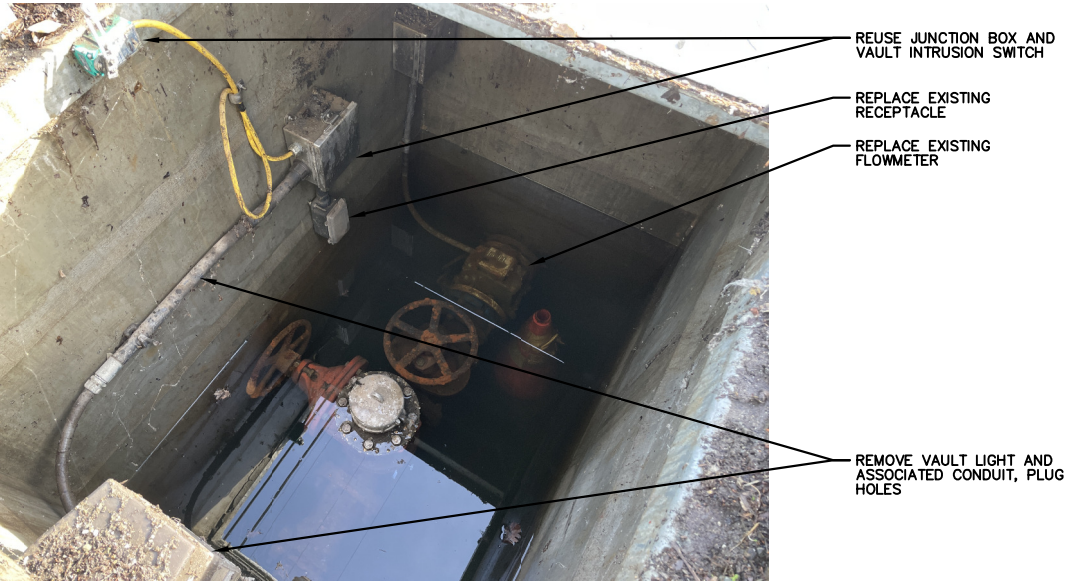
FLOWMETER VAULT PHOTO ①
