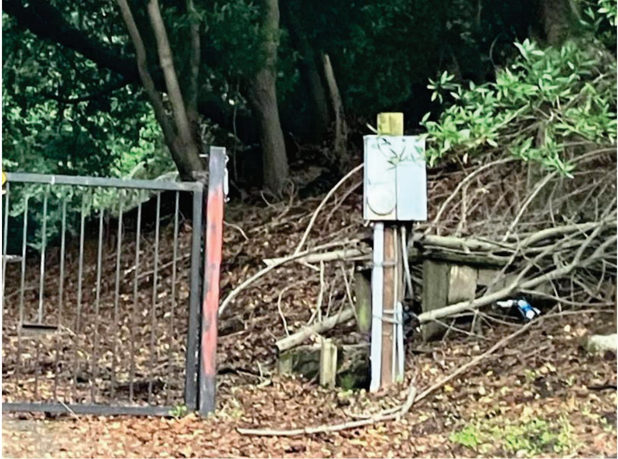
Figure 10 Breaker panel near the driveway entrance at Dublin Canyon Road, which could provide power for an electric gate on the driveway near this location
