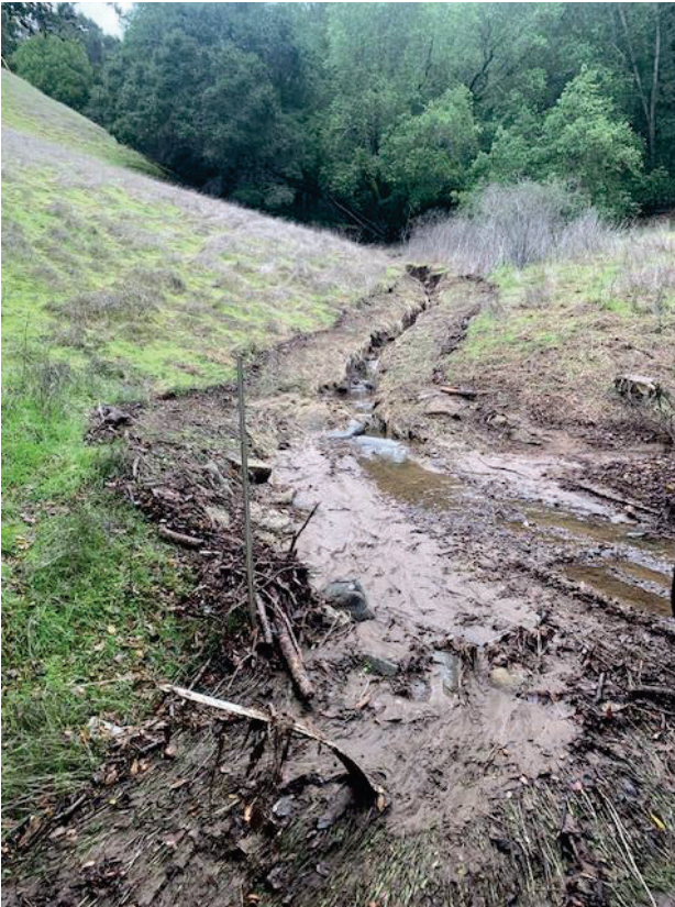
Figures 5 and 6 – Blocked Inlet Structures at Canyon 1 (above) and Canyon 2 (below)
