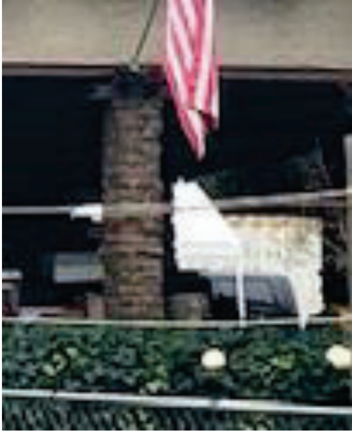
Figure 13 – Stone Column Supporting Roof Structure Over Porch. Appears to be Very Old.
