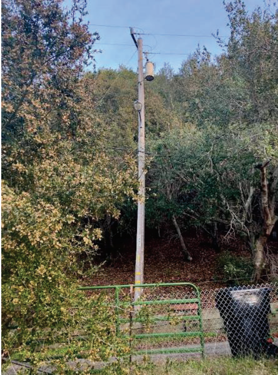
Figure 11 Street light at the driveway entrance at Dublin Canyon Road, which could provide power for an electric gate at this location
