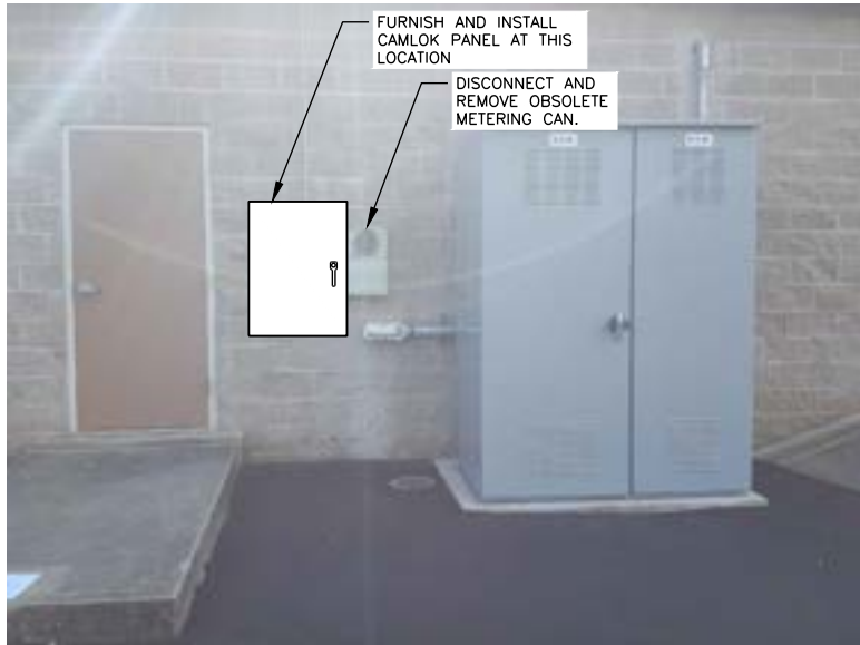
B LAUREL CREEK BOOSTER STATION (E) SERVICE SWITCHBOARD SCALE: NTS
