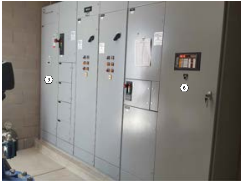
C SANTOS 900 BOOSTER STATION (E) MOTOR CONTROL CENTER SCALE: NTS
