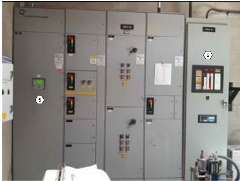
F SANTOS 1300 BOOSTER STATION (E) MOTOR CONTROL CENTER SCALE: NTS
