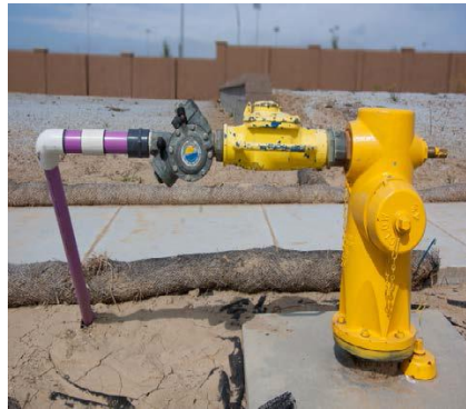
Figure 1. Acceptable temporary connection to potable fire hydrant
