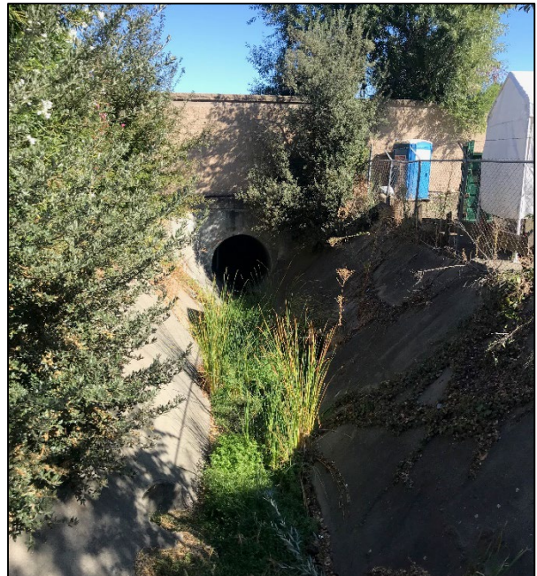
Photo 24: Stonedale Channel (C-15)
