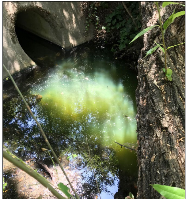
Photo 16: Standing water near culvert at Touriga Creek (C-09)
